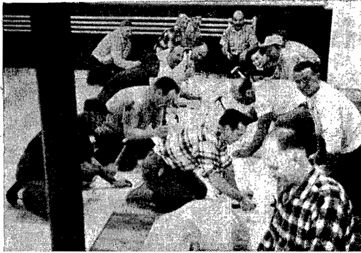
In answer to a call for help these men are laying floors at St. Mary's School. Many hours of labor have been donated and the work is progressing rapidly.
